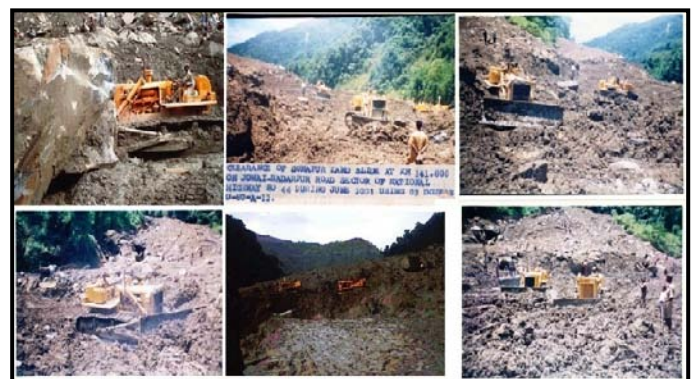
Fig. 1: Photographs of Sonapur Landslide
